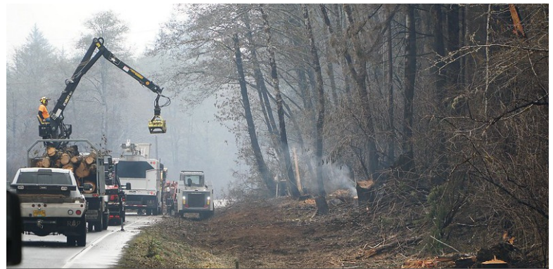
Smoke persists as crews clear out hazards on OR 18 (Credit: ODOT)
